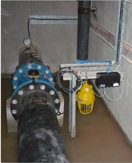
Under the ground – inside of a Turnout. Installed field controller and a junction box.
